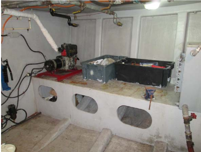
Photograph 9 - Engine room port side
