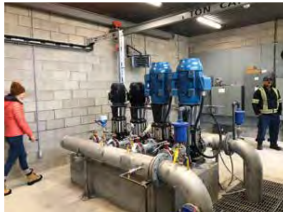
Visit by CIMA+ to Mistissini Booster Station
